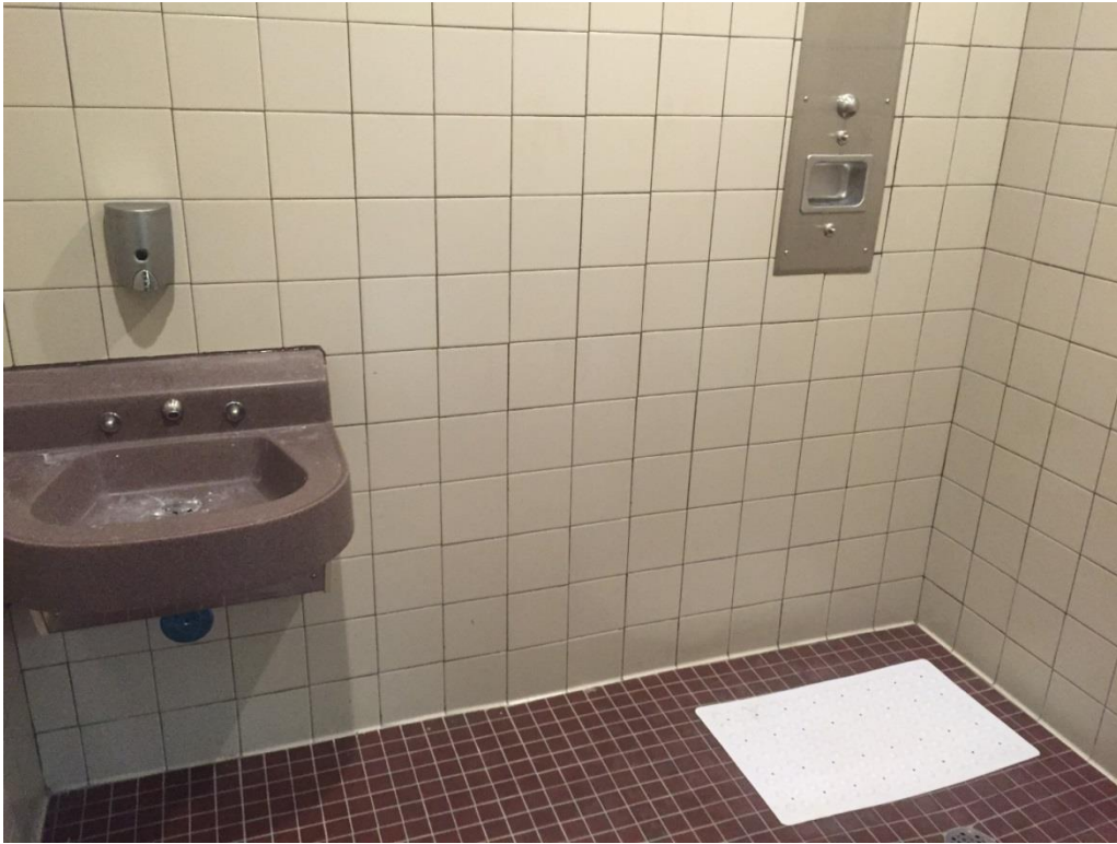
Shower and Sink Required by Texas Administrative Code
